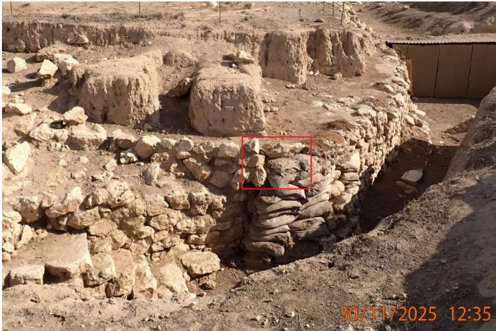
Fig. 3: Stones at risk of future collapse.
